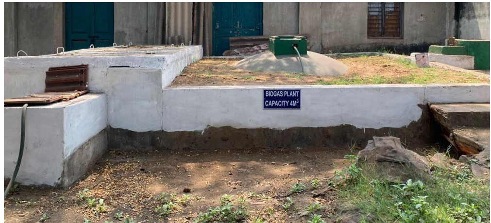
Biogas Plant at Campus
